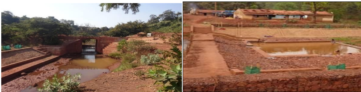
Photo Showing various Nallah protection measures undertaken outside ML
